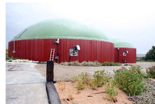
APERGAS biogas plant (Vilademuls, Girona, Spain)
